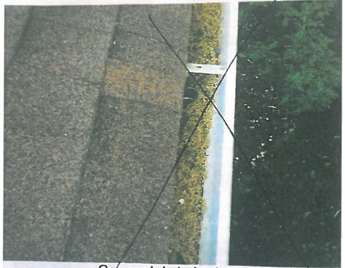
Some debris in the gutters.
