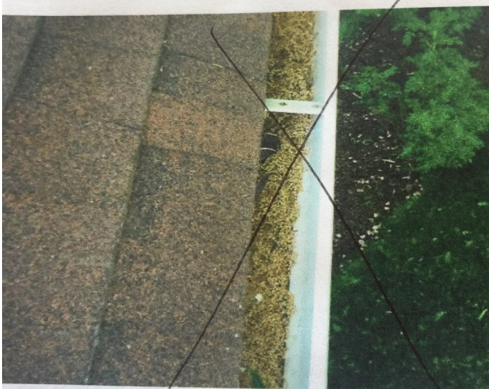
Some debris in the gutters.
